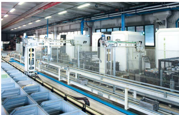
Overview of the cleaning department: last year, Ottoman implemented 3 KP 200 HMA systems from IFP Europe.
